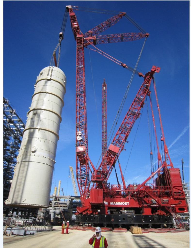
Photo of typical usage and setup for a Mammoet PTC35 ring crane (photo courtesy of Mammoet)
